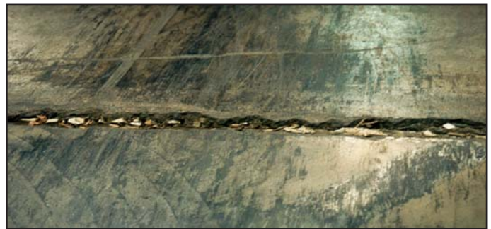
Joint deterioration is gradual but inevitable when an inferior filler is chosen or if a filler is installed poorly. As the deterioration increases, the cost of repairs increase and your productivity decreases.
